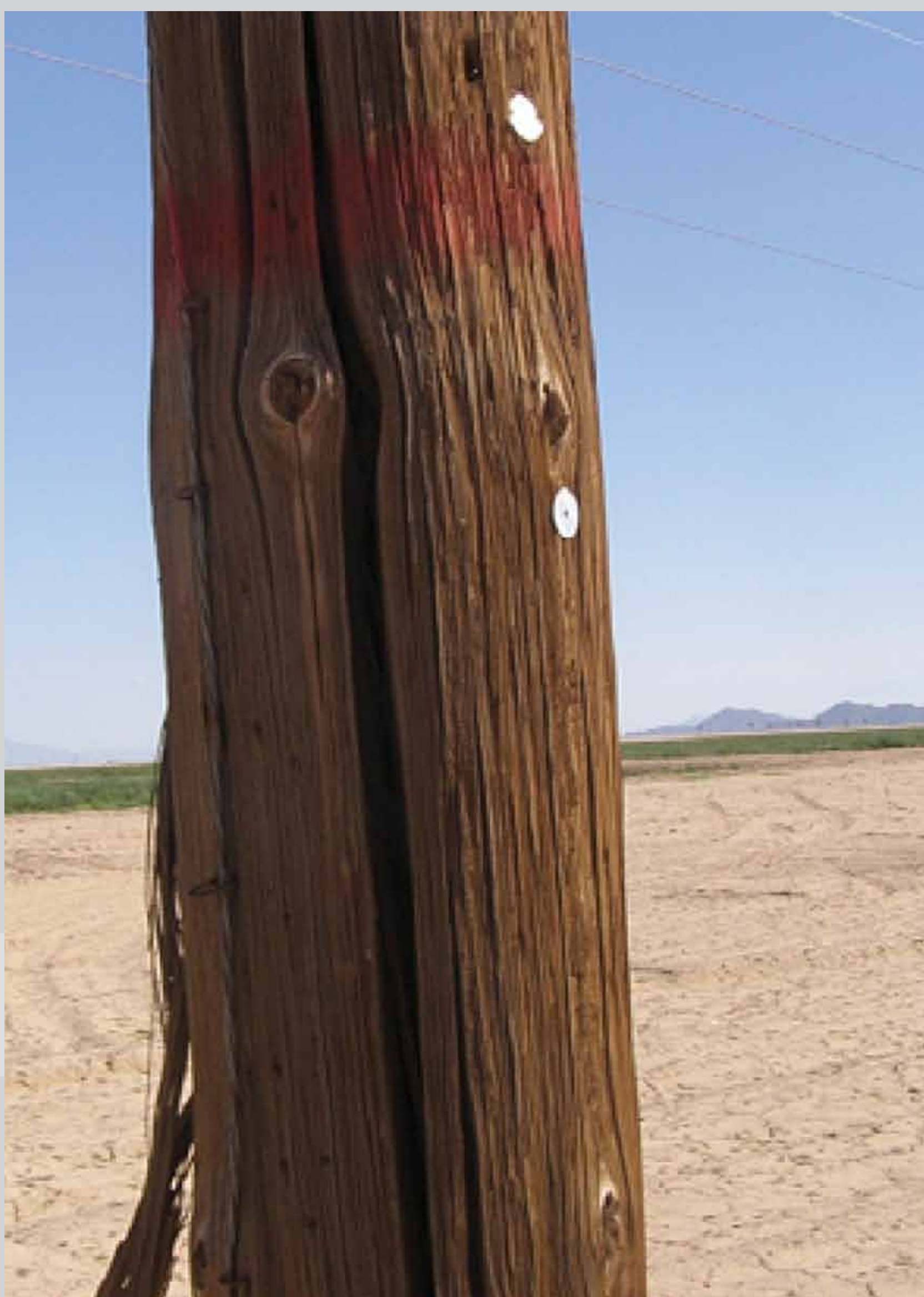
Cracked 115-kV wood pole South of Phoenix Credit: Western Area Power Administration FY2011 Ten Year Capital Program Meeting PowerPoint
