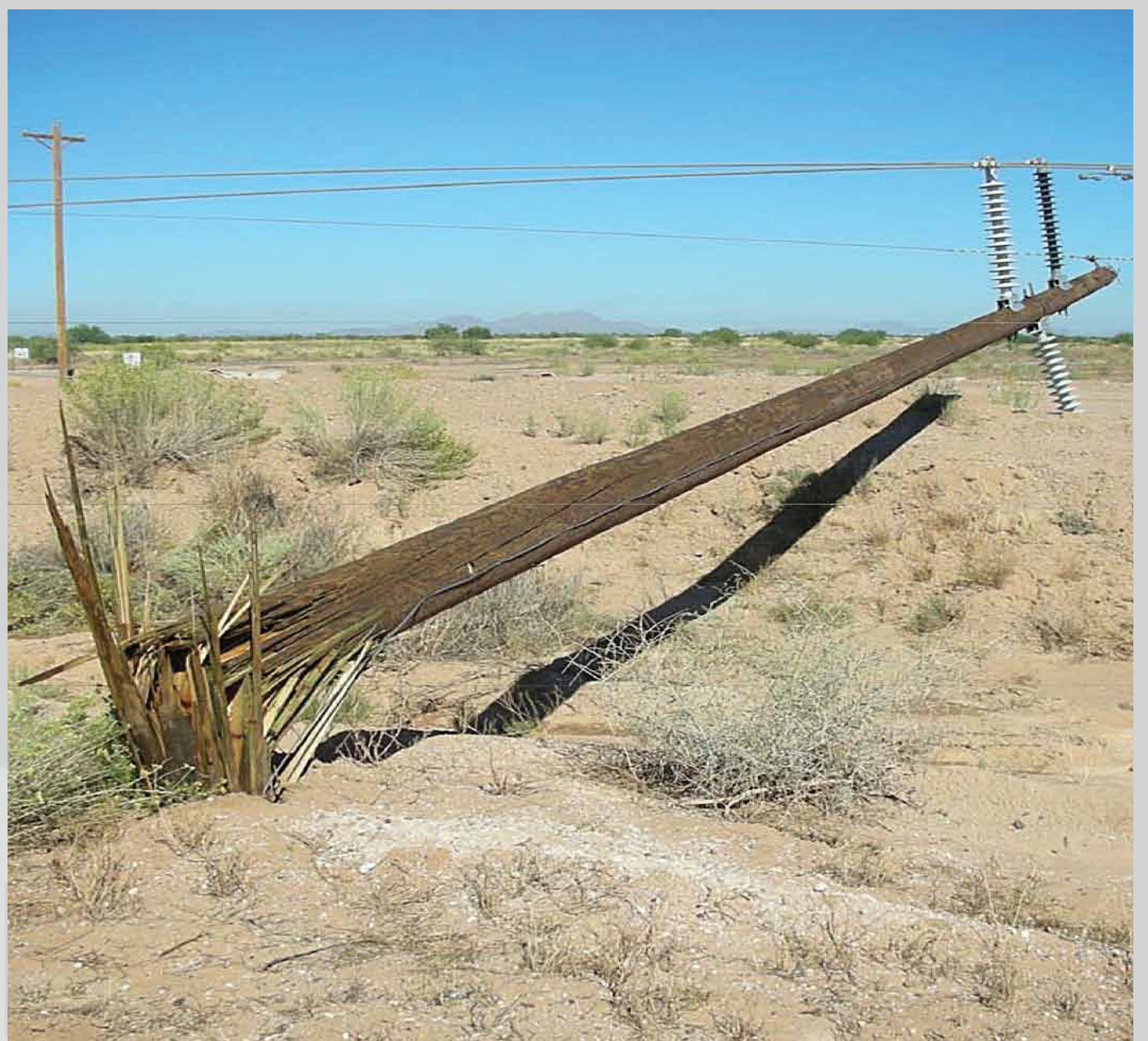
Transmission line storm damage Credit: Western Area Power Administration FY2011 Ten Year Capital Program PowerPoint
