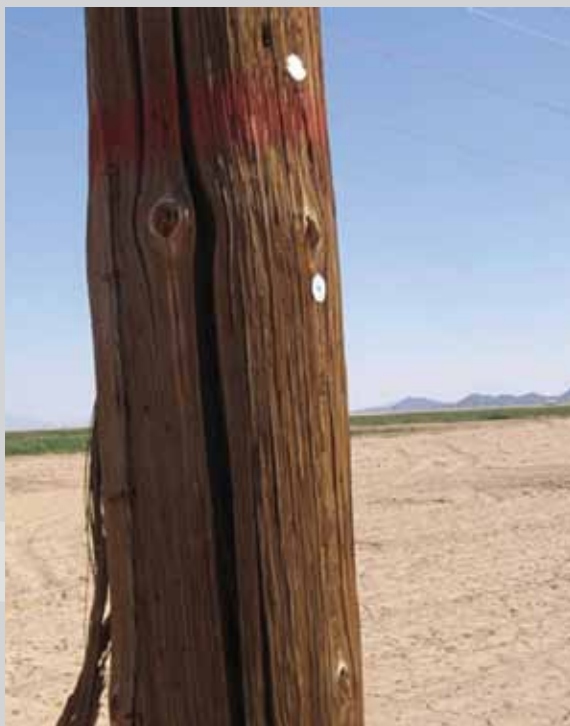
Cracked 115-kV wood pole South of Phoenix Credit: Western Area Power Administration FY2011 Ten Year Capital Program Meeting PowerPoint
